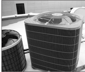
Air conditioning systems
